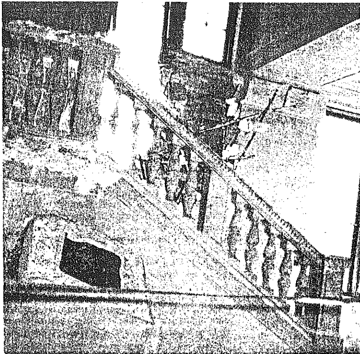
Square cement piece from fallen tower crashed through several floors and is imbedded in the marble floor in the lobby. . .
